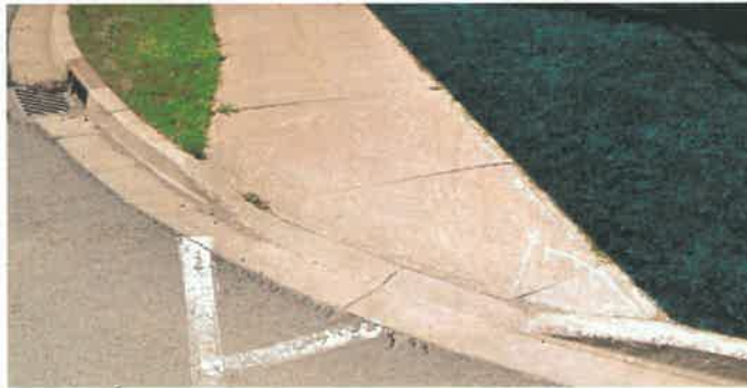
Curb ramp wider than the curb edge
