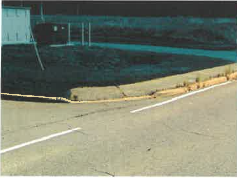
Curb ramp with cracks
