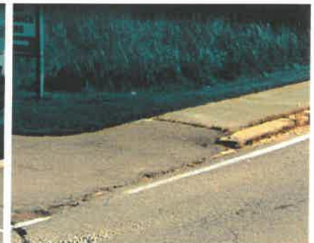
Uneven surface and withered curb edges
