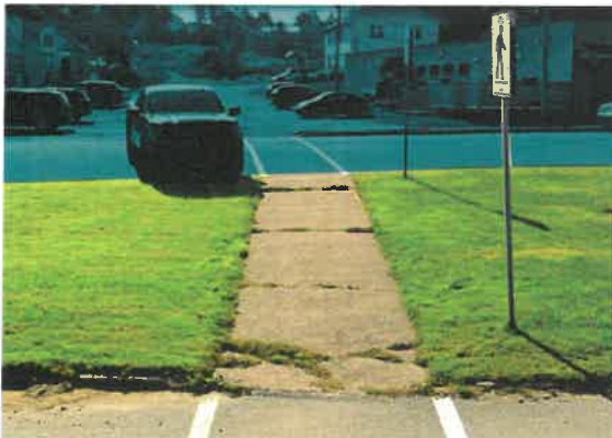
Median crossing with uneven surface
