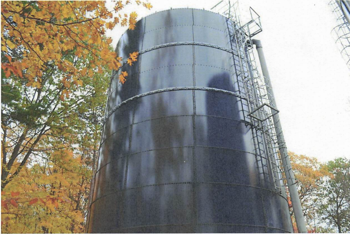
Figure 3-4: Glass-lined Bolted Steel Water Storage Reservoir/Standpipe
