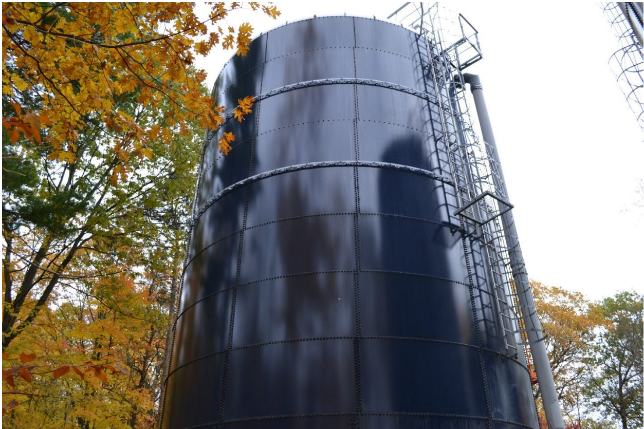
Figure 3-4: Glass-lined Bolted Steel Water Storage Reservoir/Standpipe
